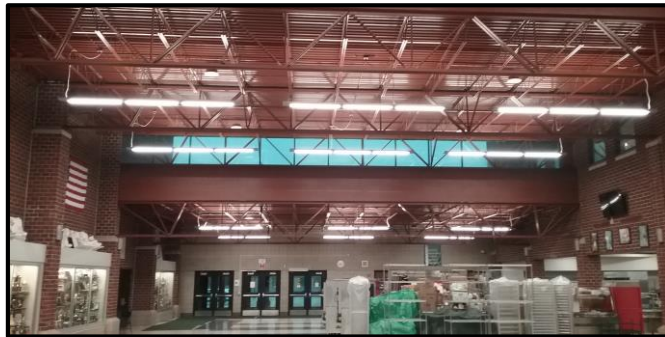
Berlin High School Commons LED Lighting
