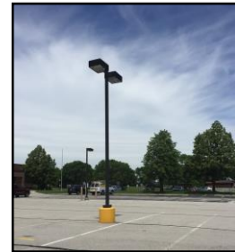
Exterior pole light - After LED Upgrade
