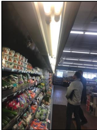
Case Lights - Before Retrofit
