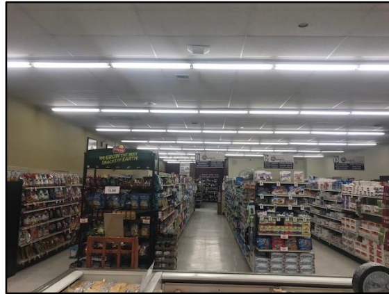
Main Isle Area lights - After Retrofit
