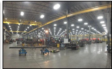
After: 18 watt LED tubes 5000K
